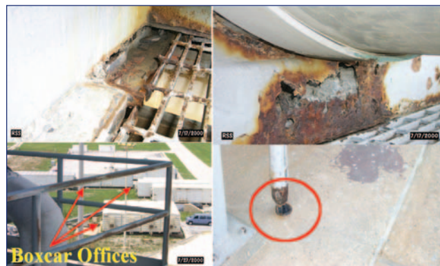
Figure 3.2.1. Launch Pad Corrosion and Boxcar Facilities.
