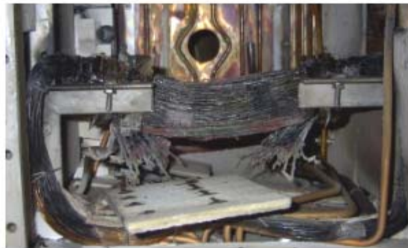
Figure 6-37 – Cable Bundle Post-Test Run #2
