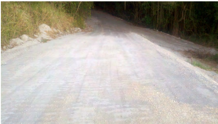
Figure 2.1 Road section with exposed AES coal ash
