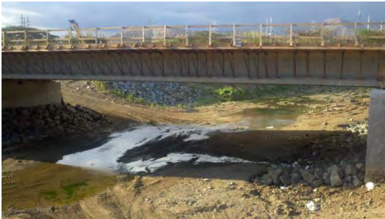
Figure 3.1 Partial view of the bridge built over the Guamaní River – south to north with AES coal ash visible in the riverbed.
