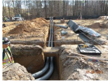
Gas lines to new energy recovery facility at Millersville Landfill
