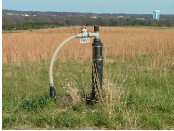
Gas Monitoring & Extraction Well
