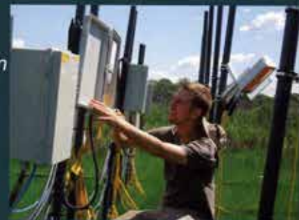
Joe Dawson checks a control box for underground heating cables
