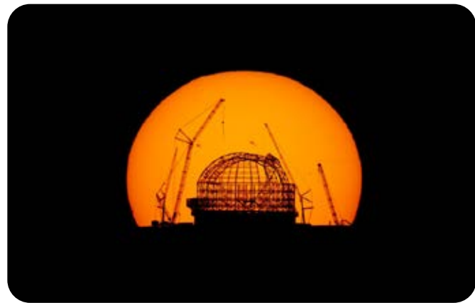
The ESO 39m Extremely Large Telescope under construction at Armazones, Chile. Image: E. Garcés/ESO. Ack.: N. Dubost
