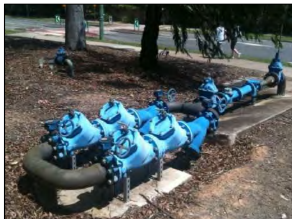
Figure 11 Culloden Road Main Meter
