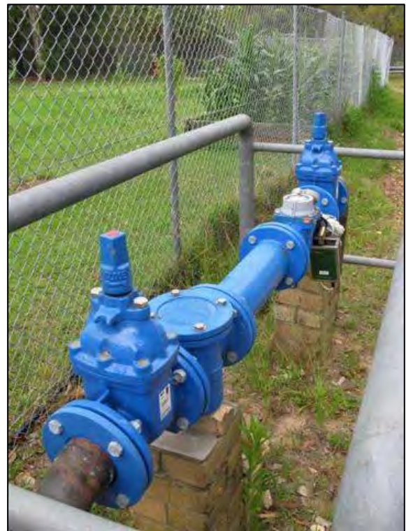
Figure 4. Sports Fields Main Meter
