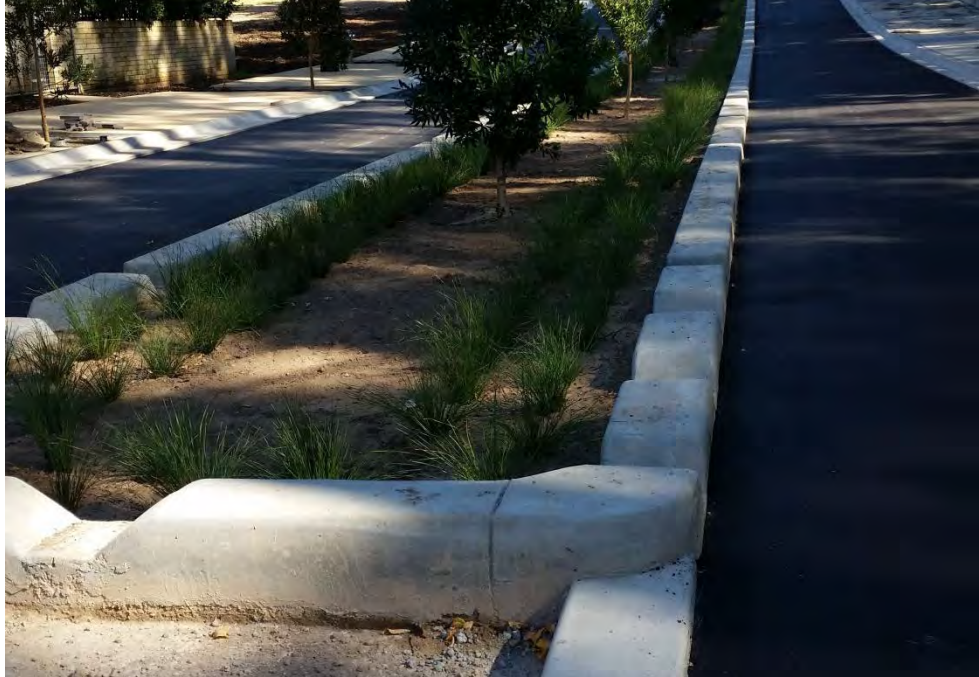
Figure 21 "Castellated kerb" allows water into the central median where it is "polished" by vegetation and slowed from entering the stormwater system. Planting benefits by being passively watered.
