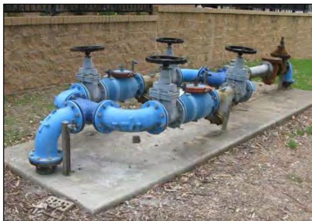
Figure 10 Balaclava Rd Main Meter
