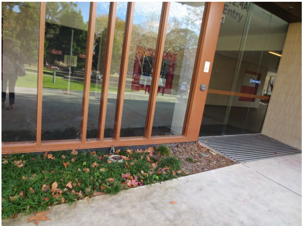
Figure 38 Mondo Grass bed requiring replacement planting
