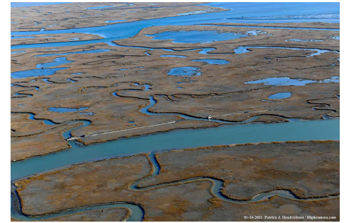
Fiber duct drilling across Wallops Island marshland. (Photo courtesy Patrick J. Henderson)
