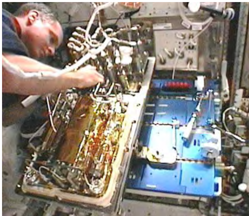
NASA's WPA Catalytic Reactor (A crew member removes the white cover in orbit to check the leaking point discovered in March 2010.)
