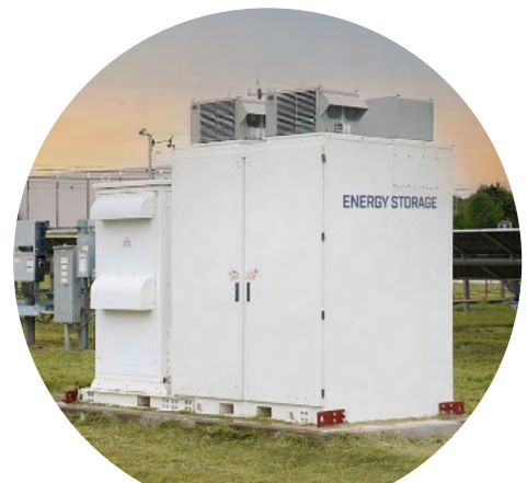
This new JIP will utilize grid-connected energy storage at SwRI's San Antonio location.
