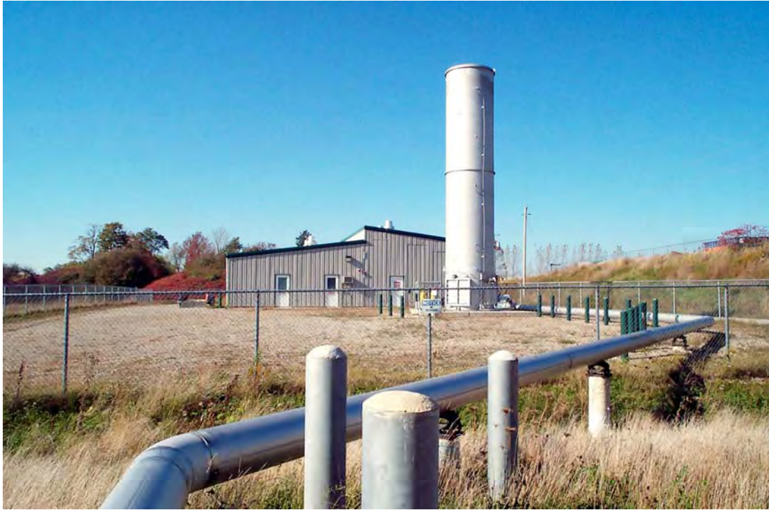
Photo 14: Enclosed Flare and Header to Landfill Gas Utilization Facility
