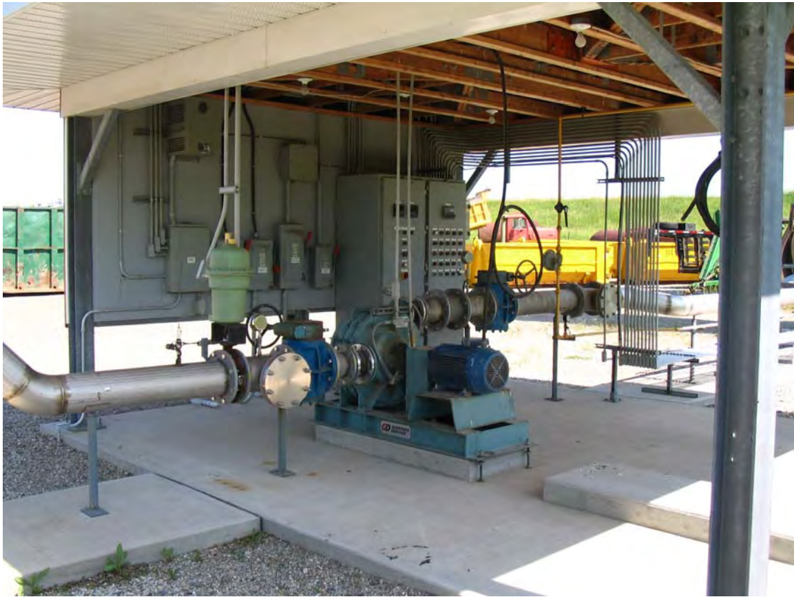
Photo 9: Landfill Gas Blower and Control Valves
