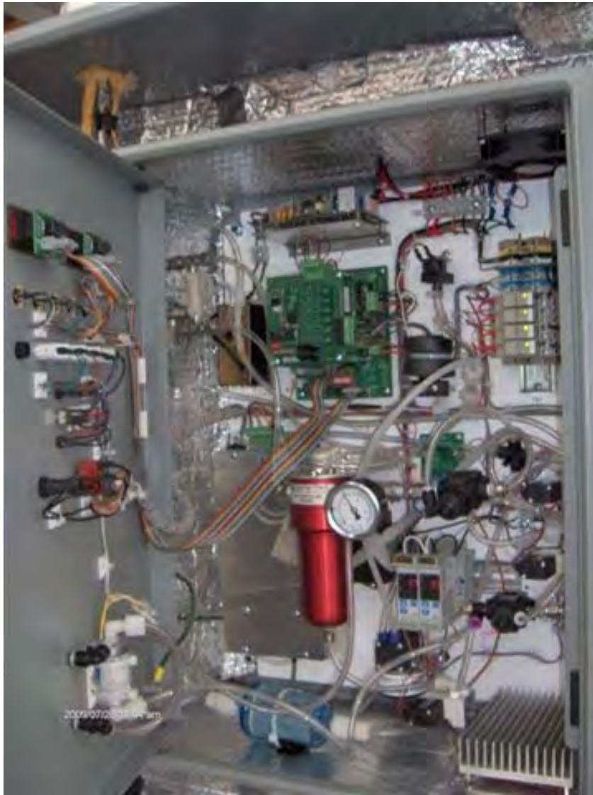
Photo 8: Inside of Landfill Gas Analyzer
