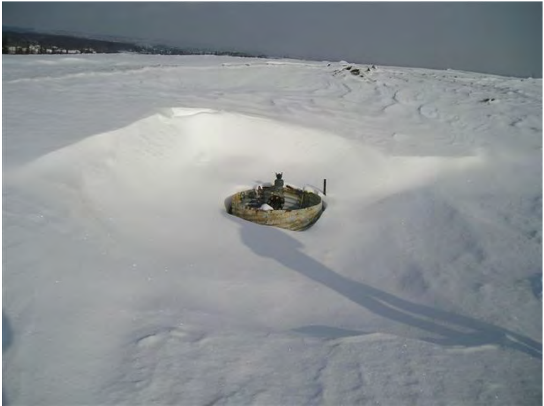
Photo 1: Vertical Landfill Gas Extraction Wellhead in Above-Ground Chamber
