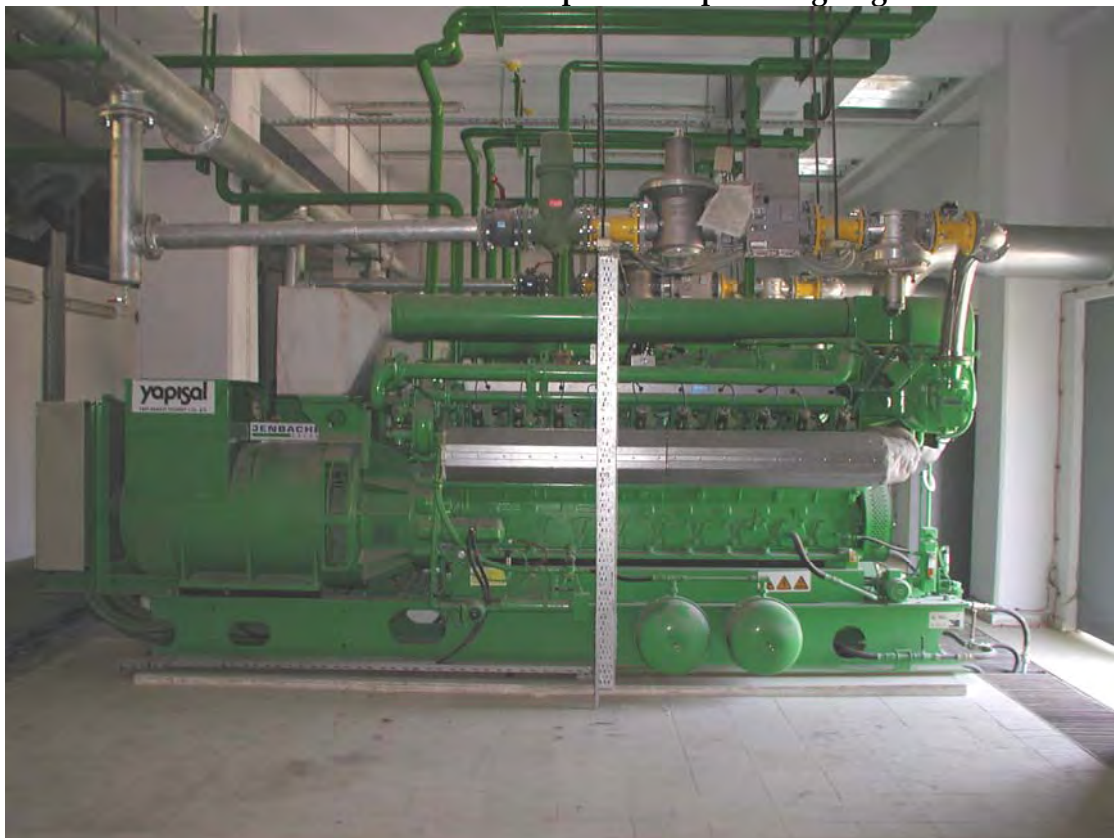
Photo 16: Example of a Jenbacher Engine (Conestoga-Rovers & Associates, 2004)
