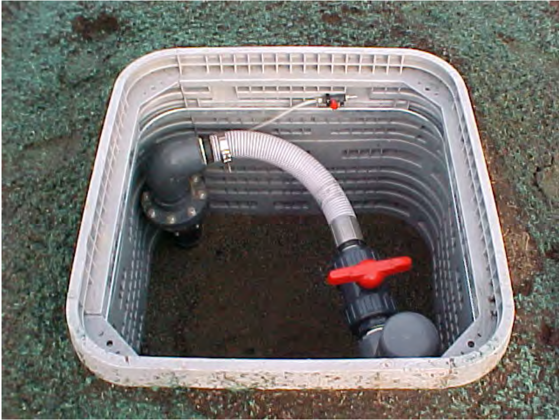
Photo 4: Typical Vertical Landfill Gas Extraction Wellhead in Below-Ground Chamber
