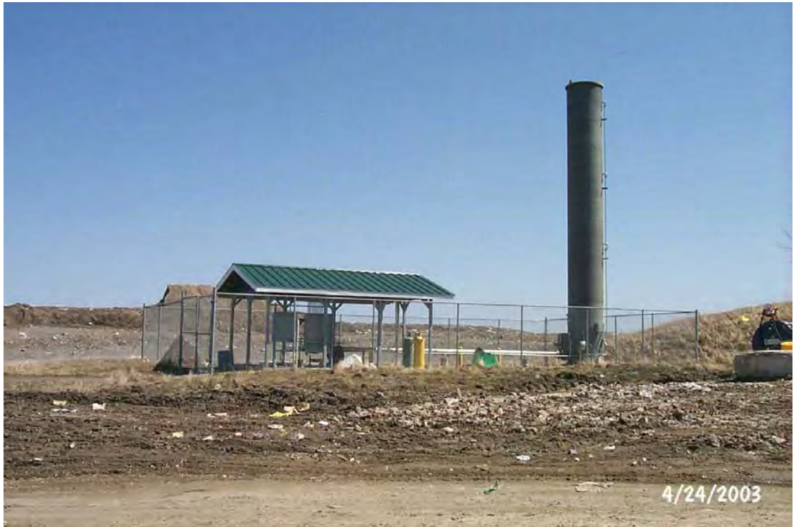
Photo 11: Landfill Gas Blower Shelter and Enclosed Flare
