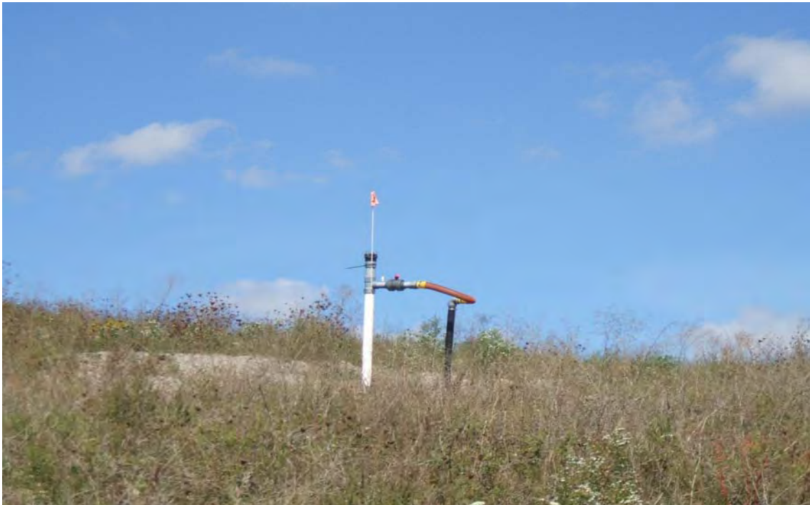
Photo 5: Typical Vertical Landfill Gas Extraction Well Stick-up
