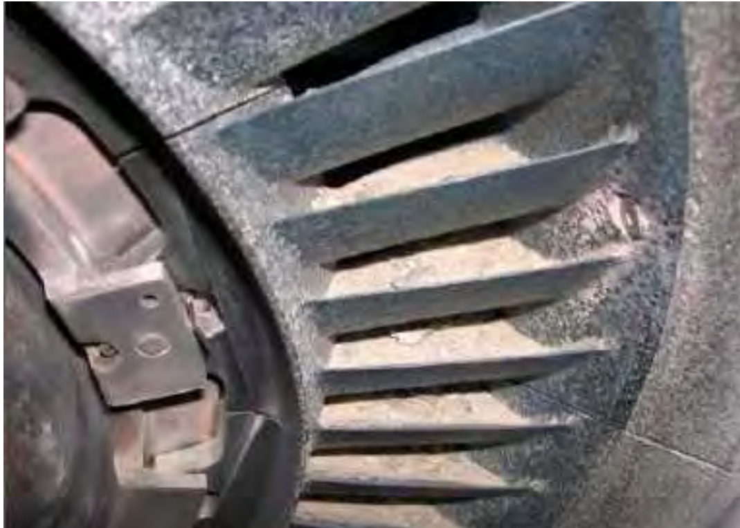
Photo 13: Siloxane deposits on turbine blade (U.S. EPA, 2006)
