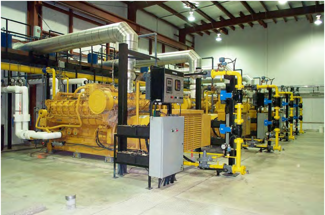
Photo 15: Landfill Gas Caterpillar Reciprocating Engines
