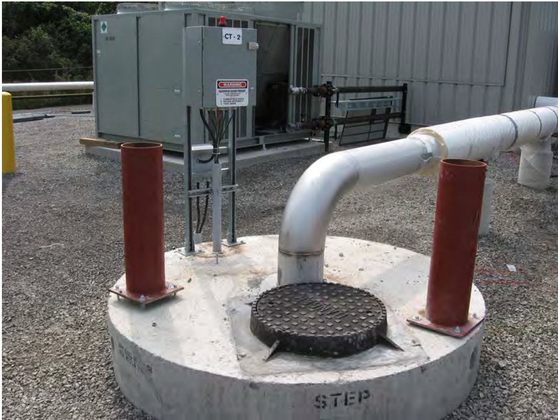
Photo 7: Condensate Trap Manhole
