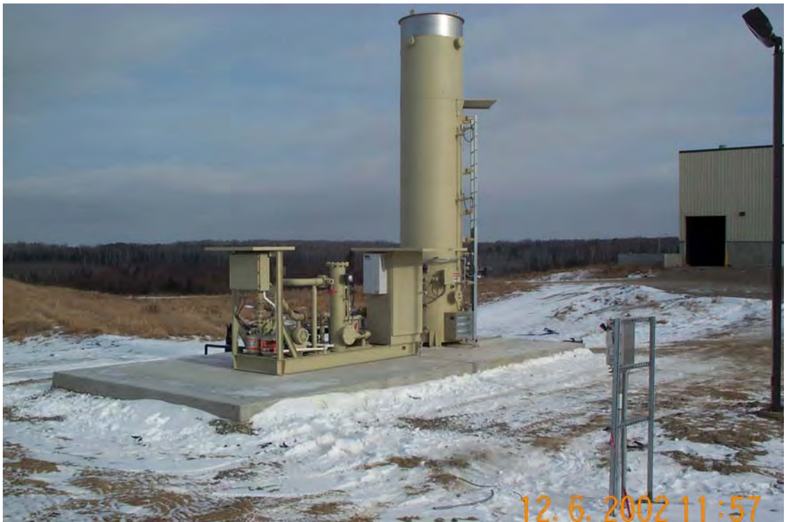
Photo 10: Skid-Mounted Landfill Gas Flare Package
